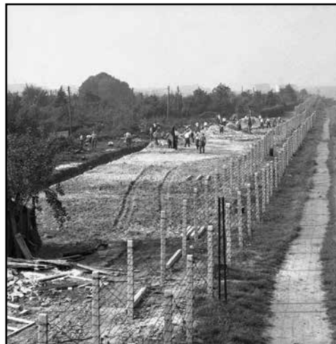
East Berlin laborers work on the "Death Strip" which communist authorities created on their side of the border in the divided city on Oct. 1, 1961. A double barbed wire fence marks the border, with West Berlin at right. In this view of the area on September 23 laborers level rubble of houses which, just days before, stood on the site close to the border. Buildings along the 25-mile dividing line were evacuated and razed by Berlin reds to eliminate one means of escape used by East Berliners to jump to the west. — AP photo
